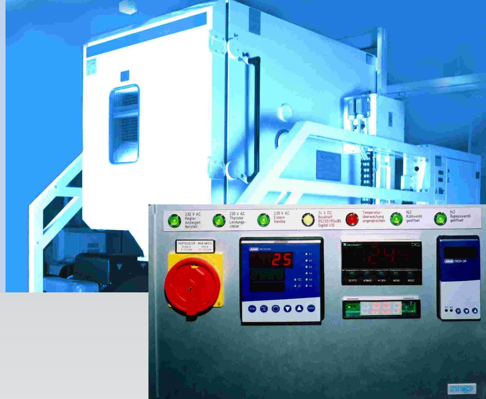
Hardware with controllers and displays in a 19" rack
