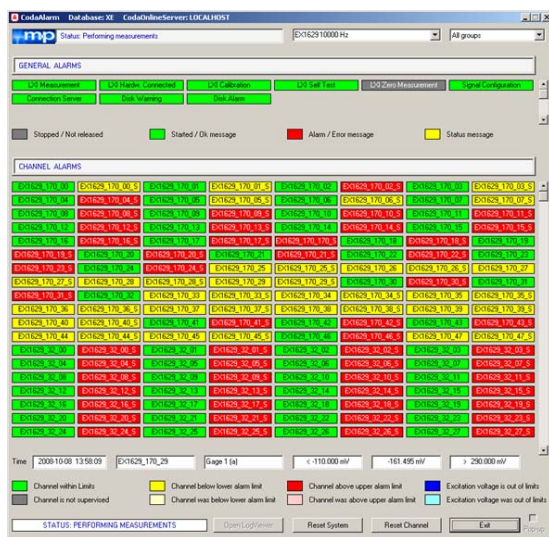
Coda alarm monitoring
